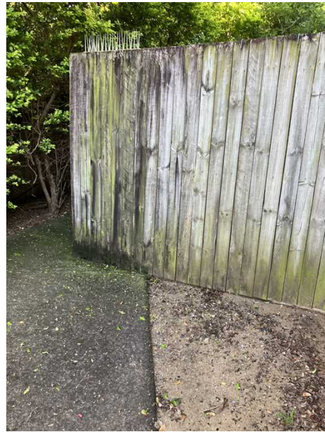
Fungal decay in timber fences
