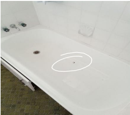
Damage to bath enamel.
