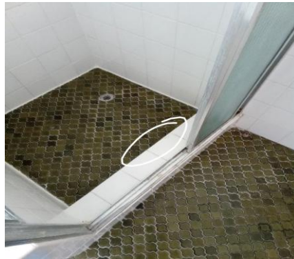
Damaged tile on hob.
