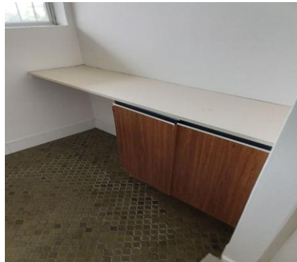
Significant deterioration due to moisture penetration.
