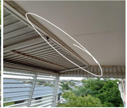
Partial detachment of timber trim.
