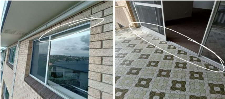
Minor surface corrosion to window lintel
