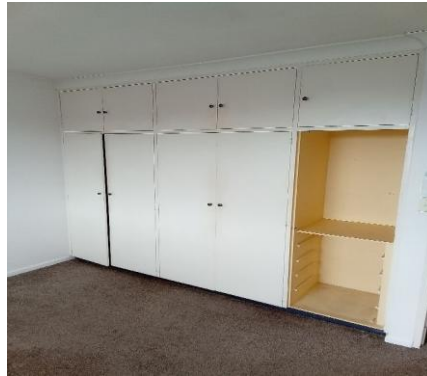
Cupboard doors binding against each other.
