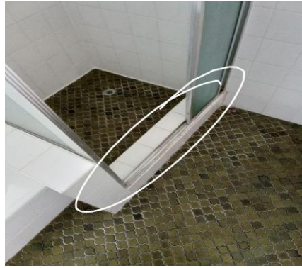
Shower screen installed inappropriately.
