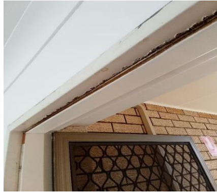
Surface corrosion to metal door frame.
