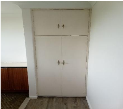
Cupboard doors binding against each other.
