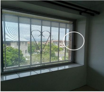
Window latch detached and missing.
