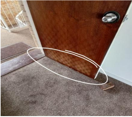
Minor deterioration to base of door.
