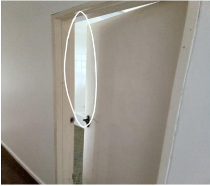
Door rubbing on frame.
