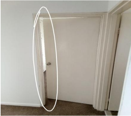
Door binding on jamb.
