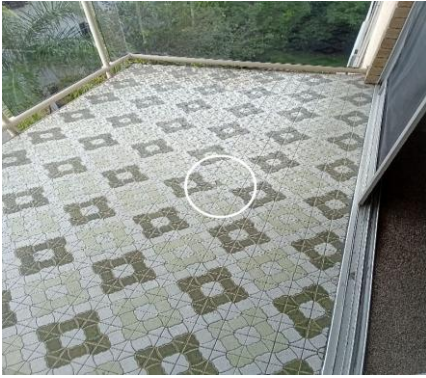
Damaged floor tile.
