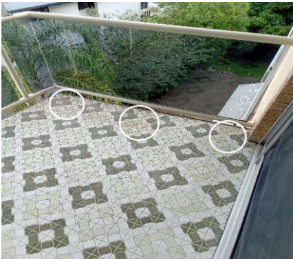
Discarded fixing holes on floor.
