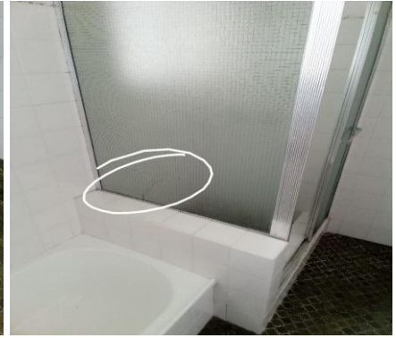
Cracked shower screen.
