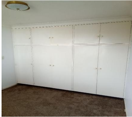
Cupboard doors binding against each other.
