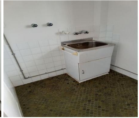
Drummy wall tiles.
