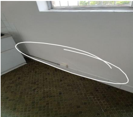
Delamination of render from base of wall.
