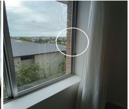
Window latches are detached and missing.
