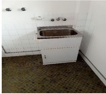
Minor surface corrosion to laundry tub.
